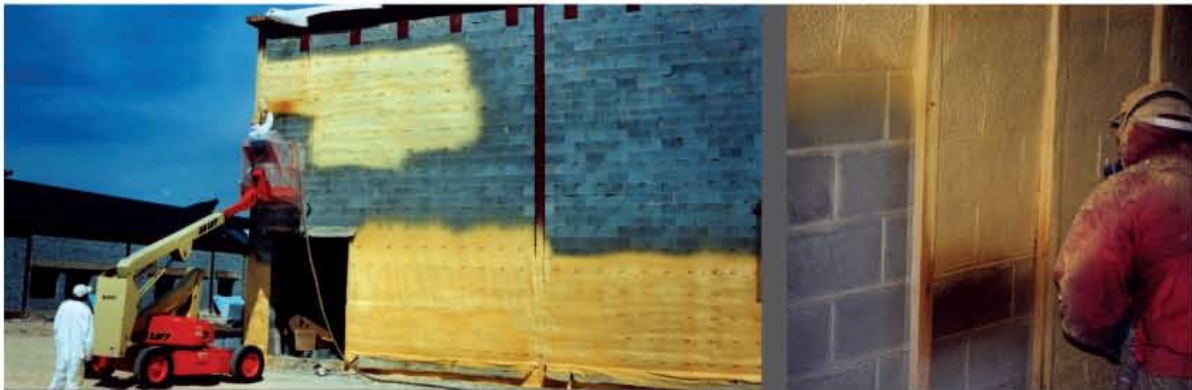
In the above curtain wall (CW) construction, 2-lb SPF is used to insulate the exterior of a building, helping to eliminate thermal bridging, while adding a secondary barrier against water penetration to the inside of the building. On the right, 2-lb SPF is used to achieve high R-value in a limited space.
